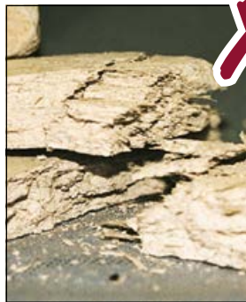
Broken asbestos insulating board
