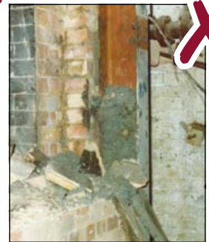
Sprayed asbestos (limpet)
